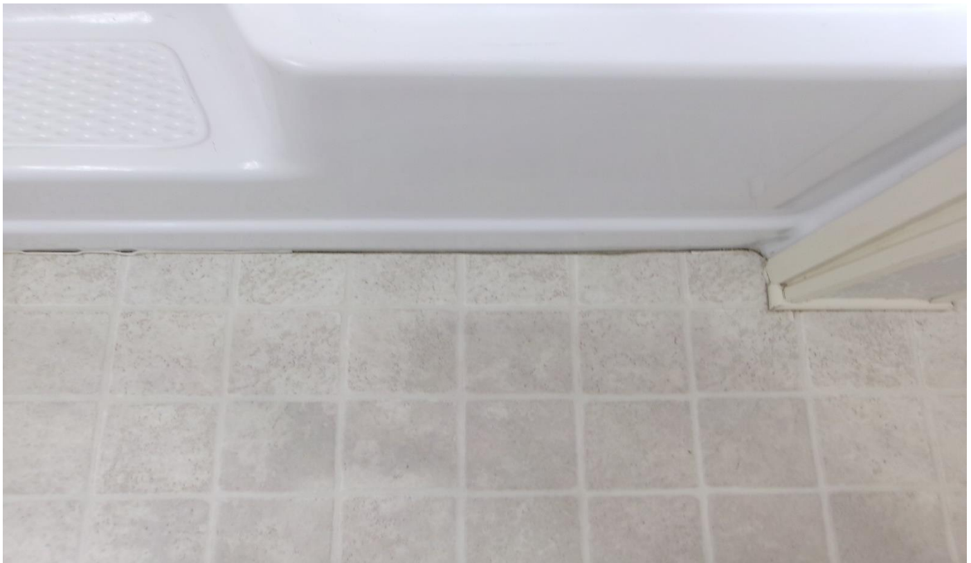
Loose / open vinyl sheet flooring at the master bathroom.
