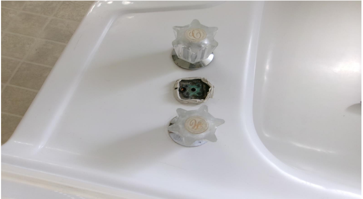
Master bathroom tub faucet has been removed.
