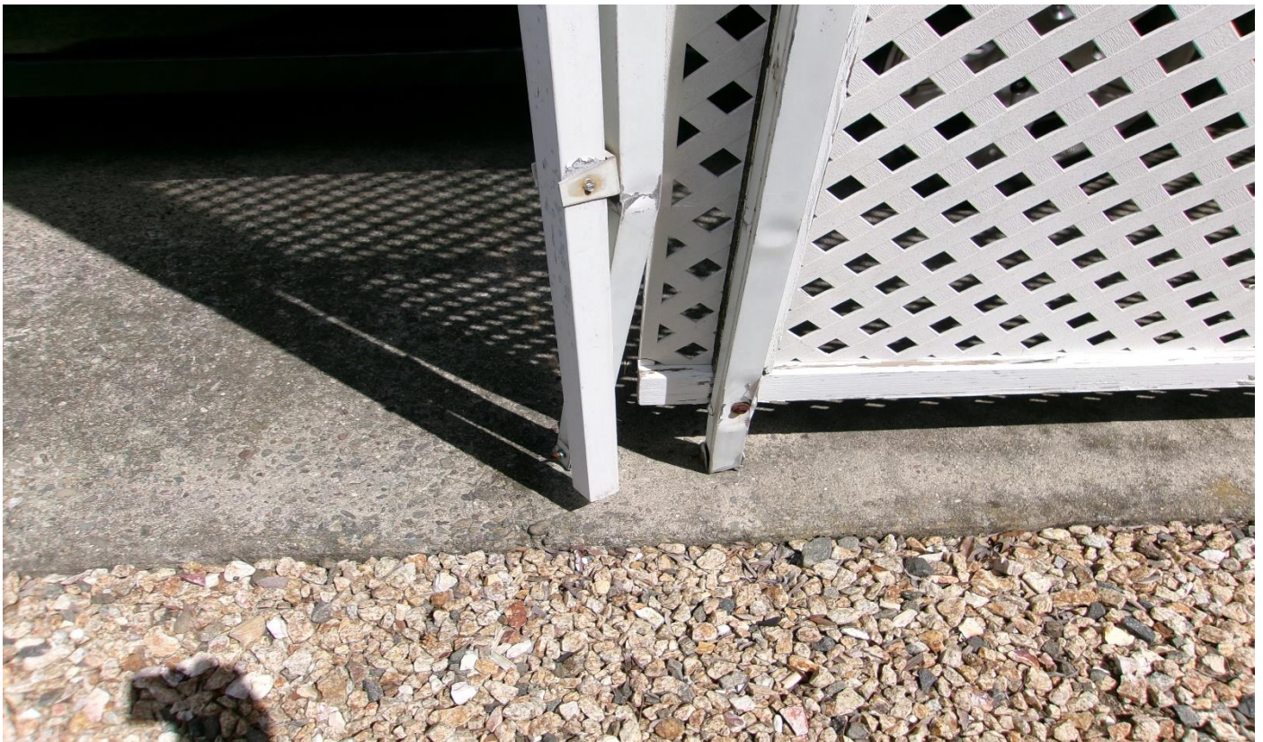
Damaged #1 carport support post.
