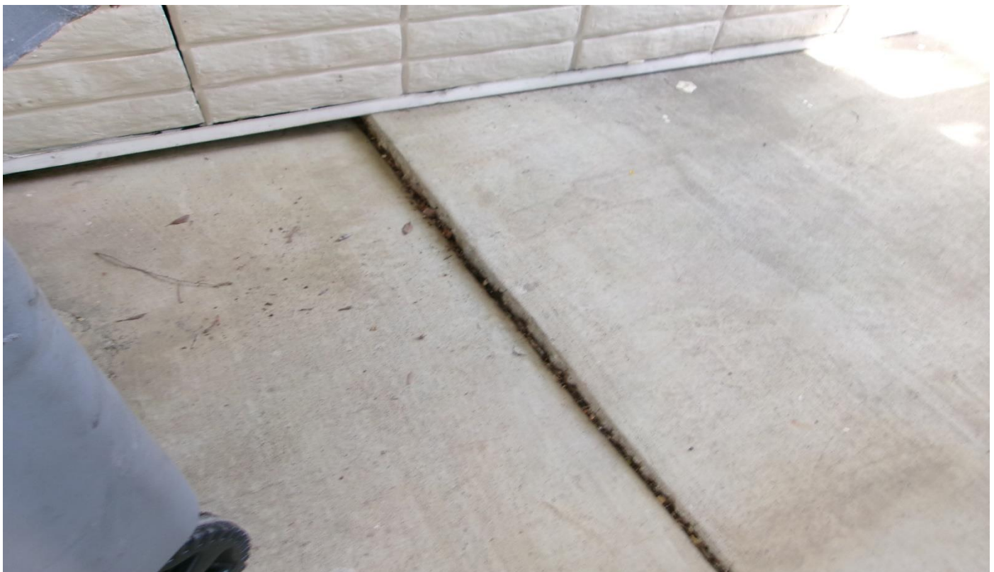
Raised concrete at the rear of the carport.
