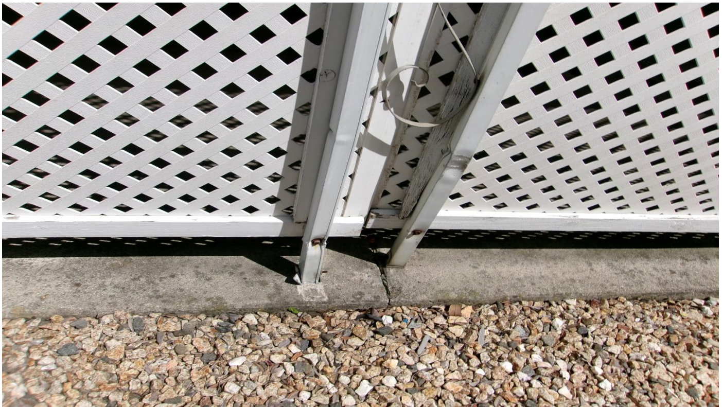
Damaged #2 carport support post.
